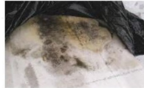
Visible mold contamination on ceiling tiles removed from room where compounding occurred.
