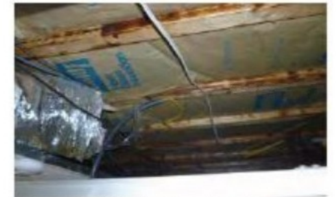
Exposed insulation in ceiling above doorway to a cleanroom.
