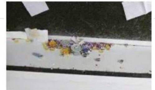
Medical supply waste and dust built up in the pre-filter of an ISO-5 hood where drugs were compounded.
